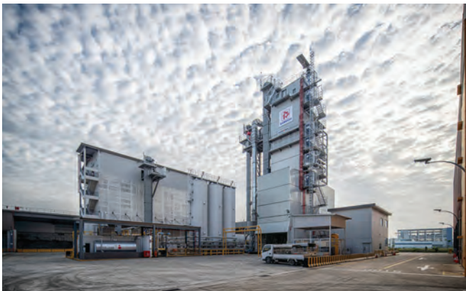
The new hub also houses Samwoh's latest asphalt production plant, which is said to be 15% more energy efficient than conventional plants and can achieve carbon abatement of 1,220 t of CO 2 per year.
