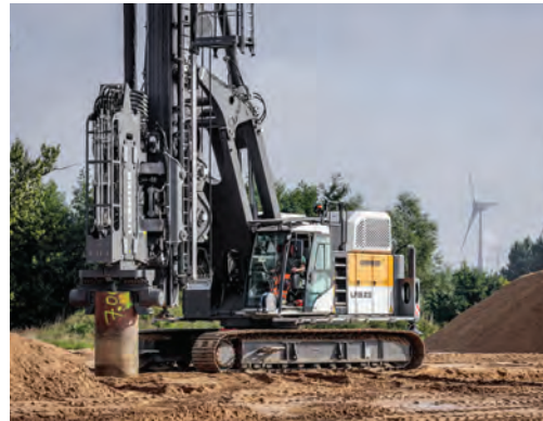
Liebherr LRB 23 piling and drilling rig (left) and HS 8070.1 duty-cycle crawler crane (below left).
